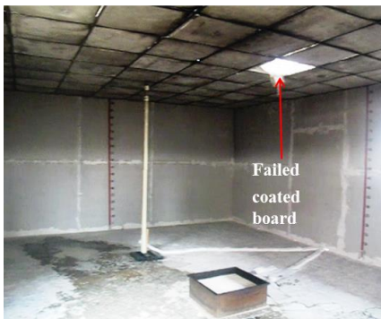
Figure 7. The failed coated board ~257 s from ignition
